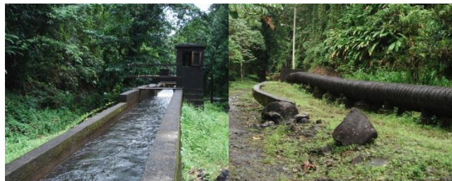
A utility-owned hydro scheme in St. Vincent and the Grenadines showing water intake infrastructure (left) and the wood-stave pipeline (right) that delivers the water to the power station turbines 59
