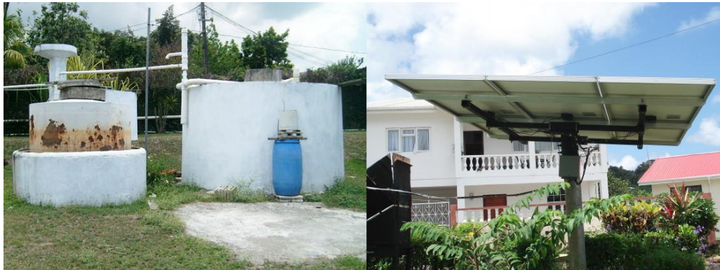
Scientific Research Council (SRC) small-scale biogas digester 100 for farms (left) and PV panels at the Grenada Chocolate Company cocoa processing factory 101
