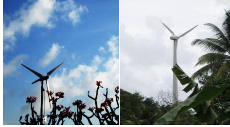
Small-scale wind-power solutions: Wind turbines installed at a private residence in St Vincent & The Grenadines (left) and at an eco-resort in Dominica 57
