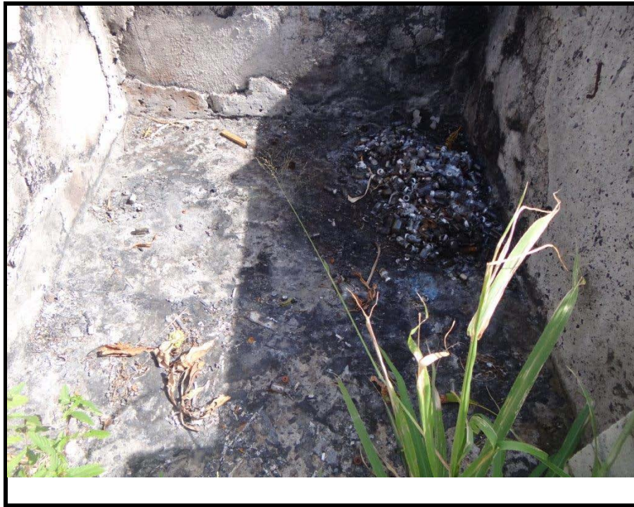
Photo 8: Concrete 'burning block' at Aitutaki District Hospital, the Cook Islands (taken 8/04/2014 by Geoff Latimer ref:DSC04146)
