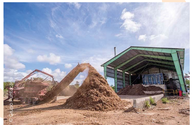
Biomass boiler, at Punta Cana Laundry Service.
