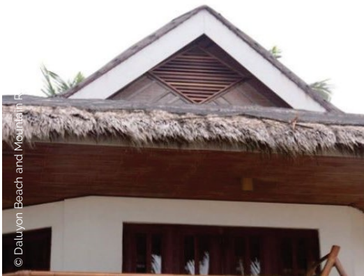
Louver ventilation installed on the roof of a guest room
