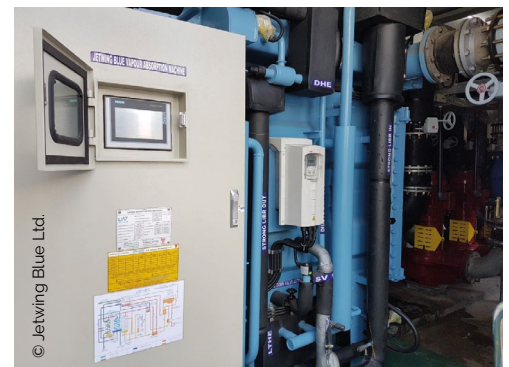
The vapour absorption chiller at Jetwing Blue
