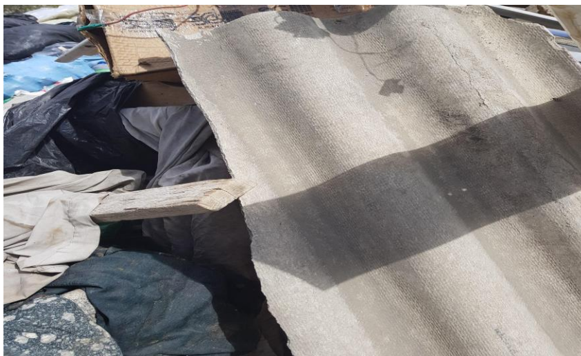
Photo 3.12 Asbestos waste, once used for roofing, is not treated with the needed security measures and ends up mixed with other waste in the environment. Photo: Nagon, 2019
