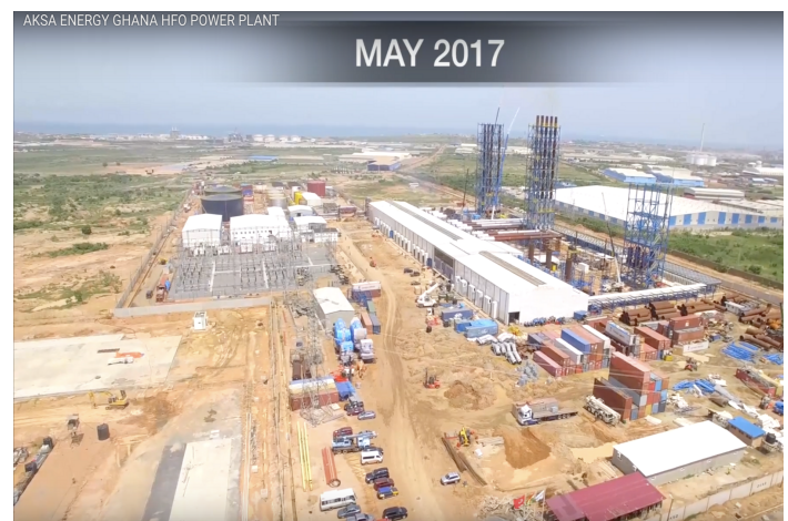
Picture 8: ASKA HFO-fired thermal power plant
