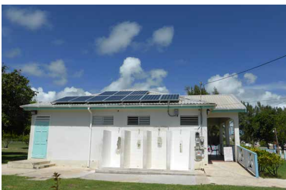
Solar Power panels on a beach facility in Silver Sands, Barbados
