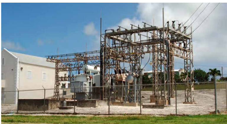
North Substation, Maynards, St Peter, Barbados
