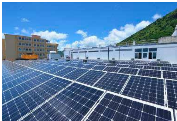
Solar panel installations in Mauritius ©UNEP
