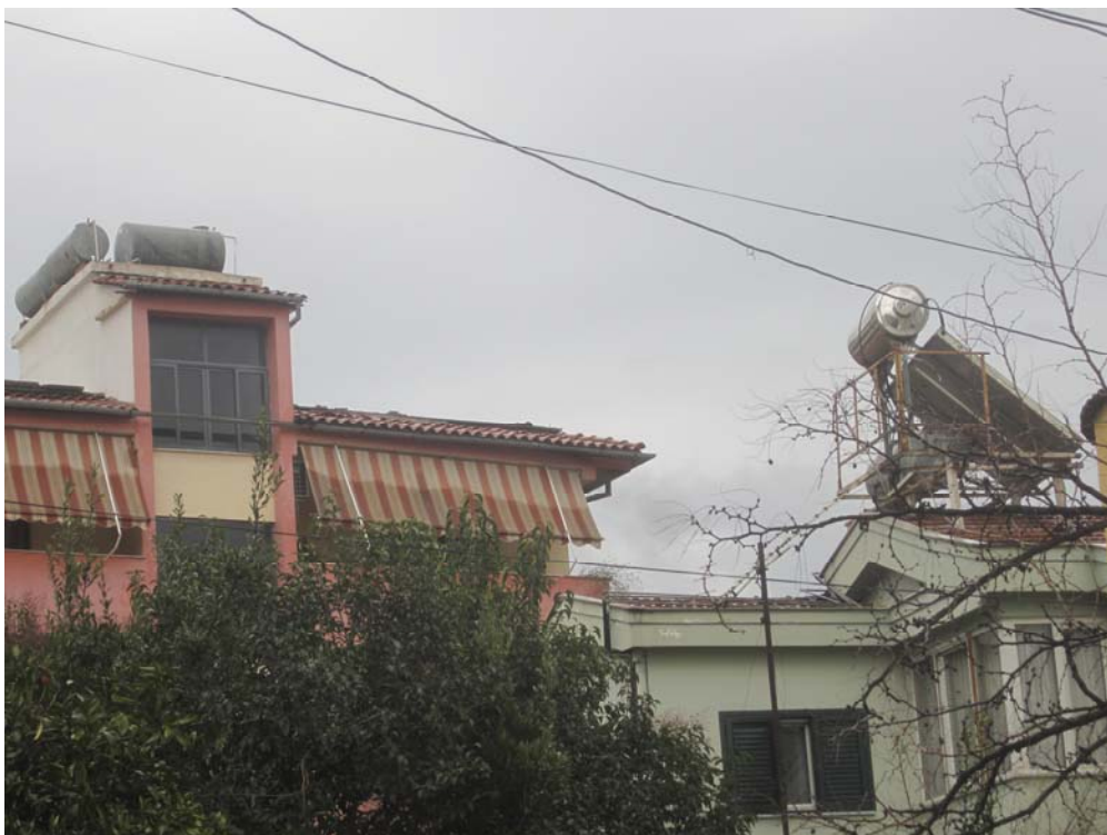
Photo 7.1: Equipment for continuous water supply
