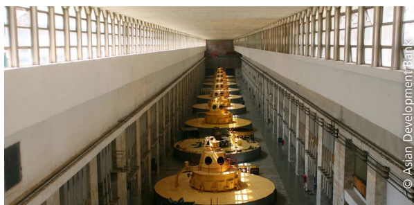
Turbines at the Nurek hydropower plant, which supplies more than 70 percent of Tajikistan's electricity.
