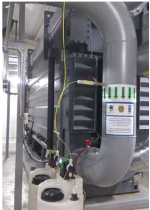
ABSORPTION REFRIGERATING MACHINE (ARM) – HEART OF THE ENERGY COMPLEX. PHOTO CREDIT: VALERY PISHCHIK
