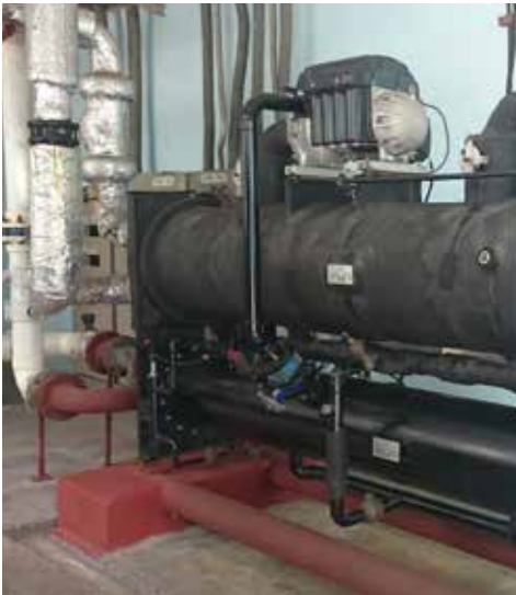
OLD AND NEW CHILLERS AT SANTA CLARA HOSPITAL. PHOTO CREDIT: CARLOS ANDRÉS HERNÁNDEZ, UNDP MPU
