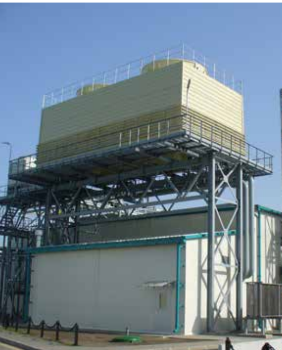
GENERAL VIEW OF ENERGY COMPLEX “SANTA BREMOR” IN BREST, BELARUS. PHOTO CREDIT: VALERY PISHCHIK
