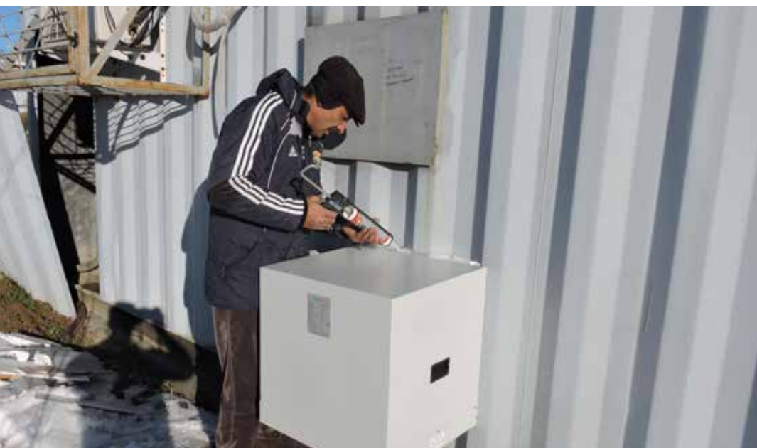
INSTALLATION OF THE ENERGY EFFICIENT COOLING MODULE AT MOBILE BASE STATION. PHOTO CREDIT: UNDP TAJIKISTAN
