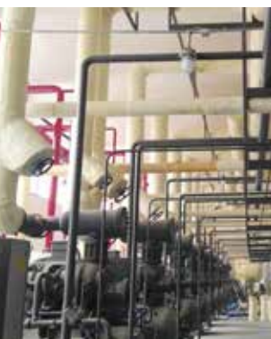
WORKSHOP OF CHINA'S LARGEST NH 3 /CO 2 REFRIGERATION SYSTEM WITH 16 SETS EACH OF NH 3 AND CO 2 COMPRESSORS. PHOTO CREDIT: YANTAI MOON GROUP CO. LTD.
