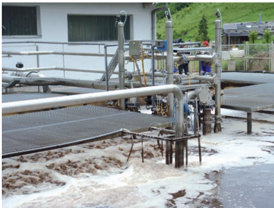
Photo 3.1: Wastewater treatment plant, Sarajevo
