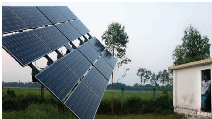
Solar powered pumps help reduce irrigation costs in Bangladesh. —Dominic Chavez/World Bank
