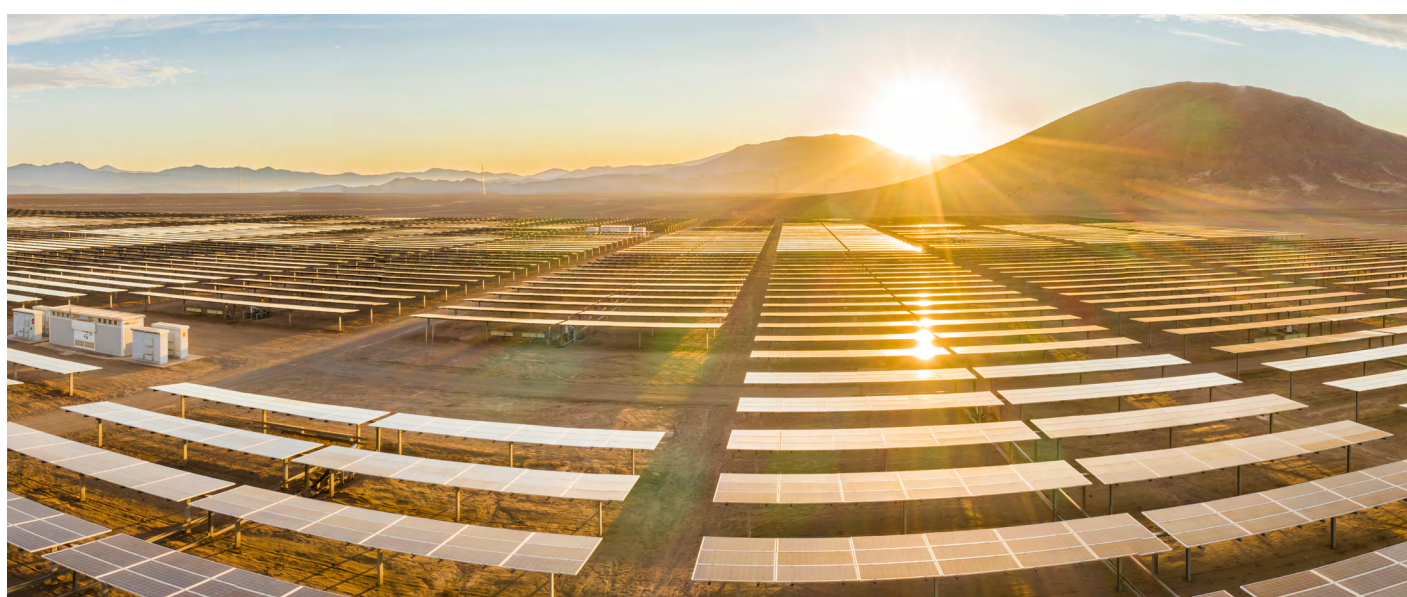
Solar Energy Photovoltaic Power Plant over Atacama desert sands, Chile
