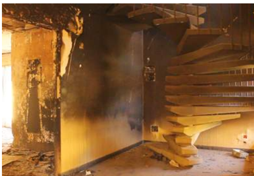
Figure 13: Fire damage to building interior
