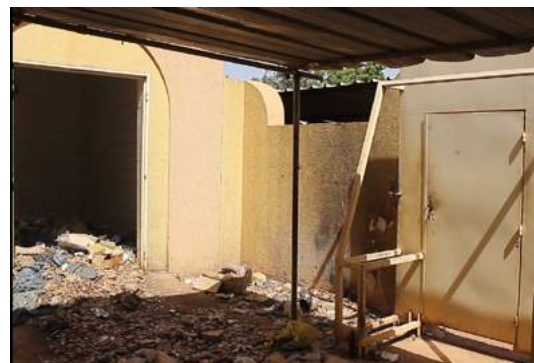
Figure 14: Vandalism and fire damage to courtyard
