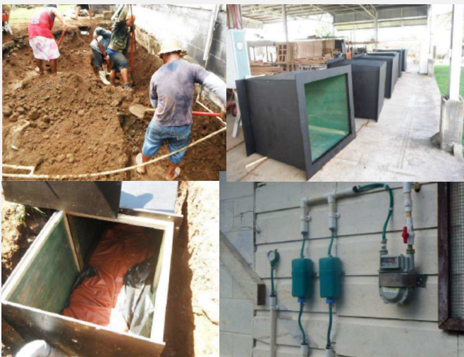
Community Biogas Reactor in Samoa – Site Preparation, Tank Modules, Biogas Bags, Gas Equipment Image Source: Ward and Rucks, 2013
