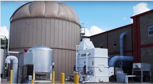
Hermitage Municipal Authority Wastewater Treatment Plant Co-Digestion Food Waste Image Source: Waste Management World, 2016
