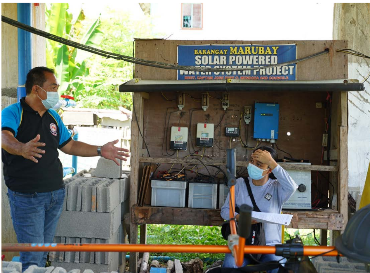
Barangay Marubay's Solar-Powered Water System. Photo from People in Need (PIN).
