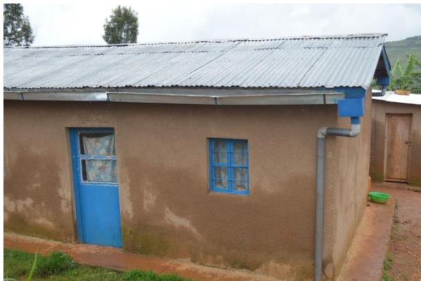
FIGURE 3-2 ROOFTOP RAINWATER HARVESTING
